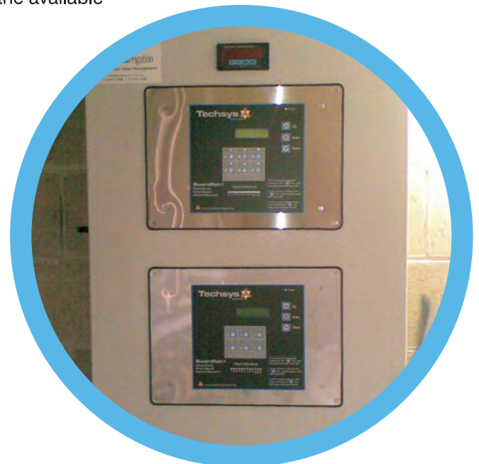
The custom designed panel controls and monitors the system
