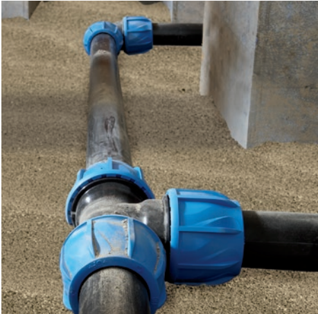
Water Distribution Lines
